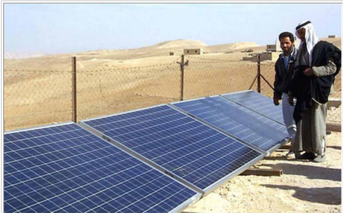
Leaders of Al-Kaabneh, a Bedouin village in the West Bank, survey the large solar power modules provided by Greenstar.
