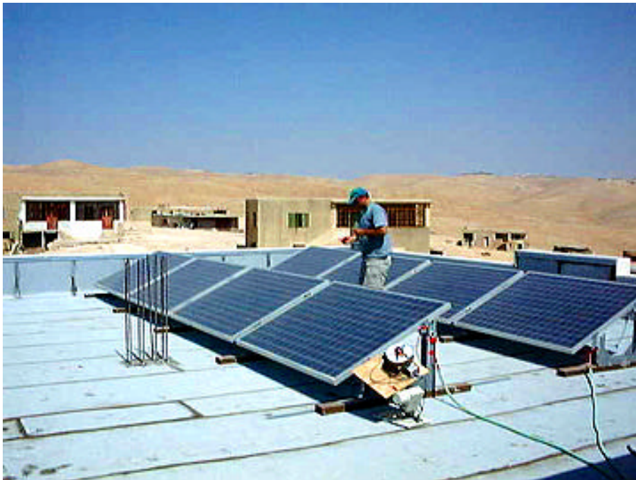
Figure 1: The roof-mounted PV array at Al Kaabneh high school. Modules shown (left to right) are: back row, “A” through “D”; front row; “E” through “H”. (See Table 1)
