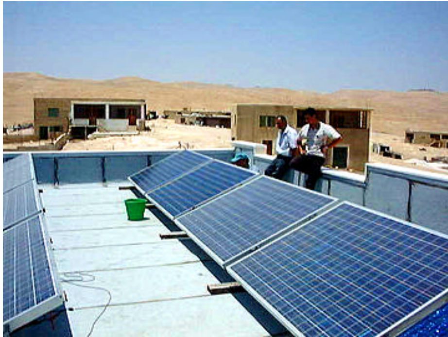
Figure 4: Modules “A” and “B” after cleaning, compared with “as is” neighboring modules
